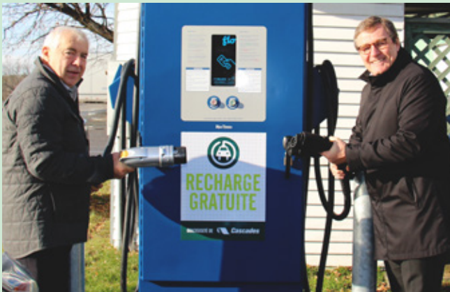
Alain Lemaire and Mario Plourde standing beside the fast charging station installed at the Cascades head office in Kingsey Falls, and made available to the community free of charge.
